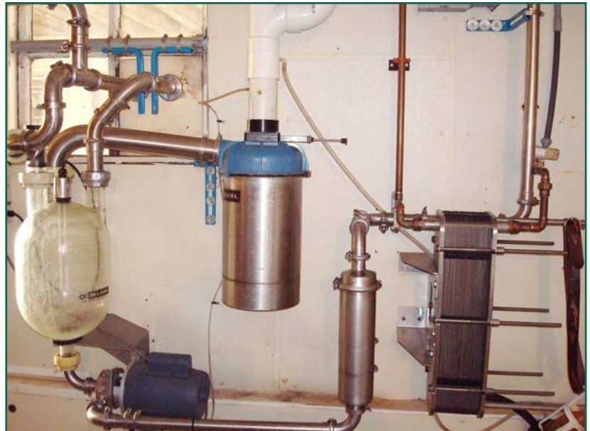
A well water precooler (far right) cuts compressor use by using groundwater to pre-cool the milk. Photo by Andy Pressman.
